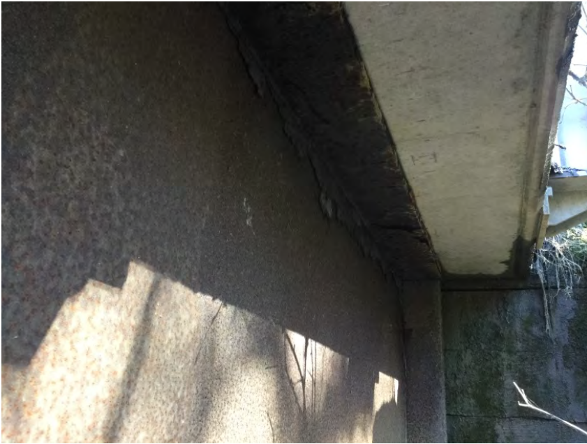
Steel delamination noted on girders
