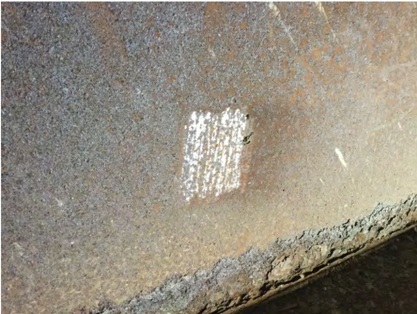
Location of previous web measurements - no further delamination
